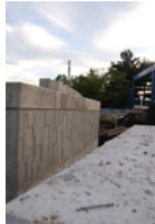
The concrete wall, pictured here, is part of gate construction, scheduled to finish in November.
